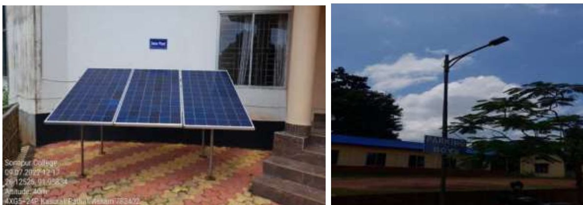
Fig. 4.3 : Solar power plant
